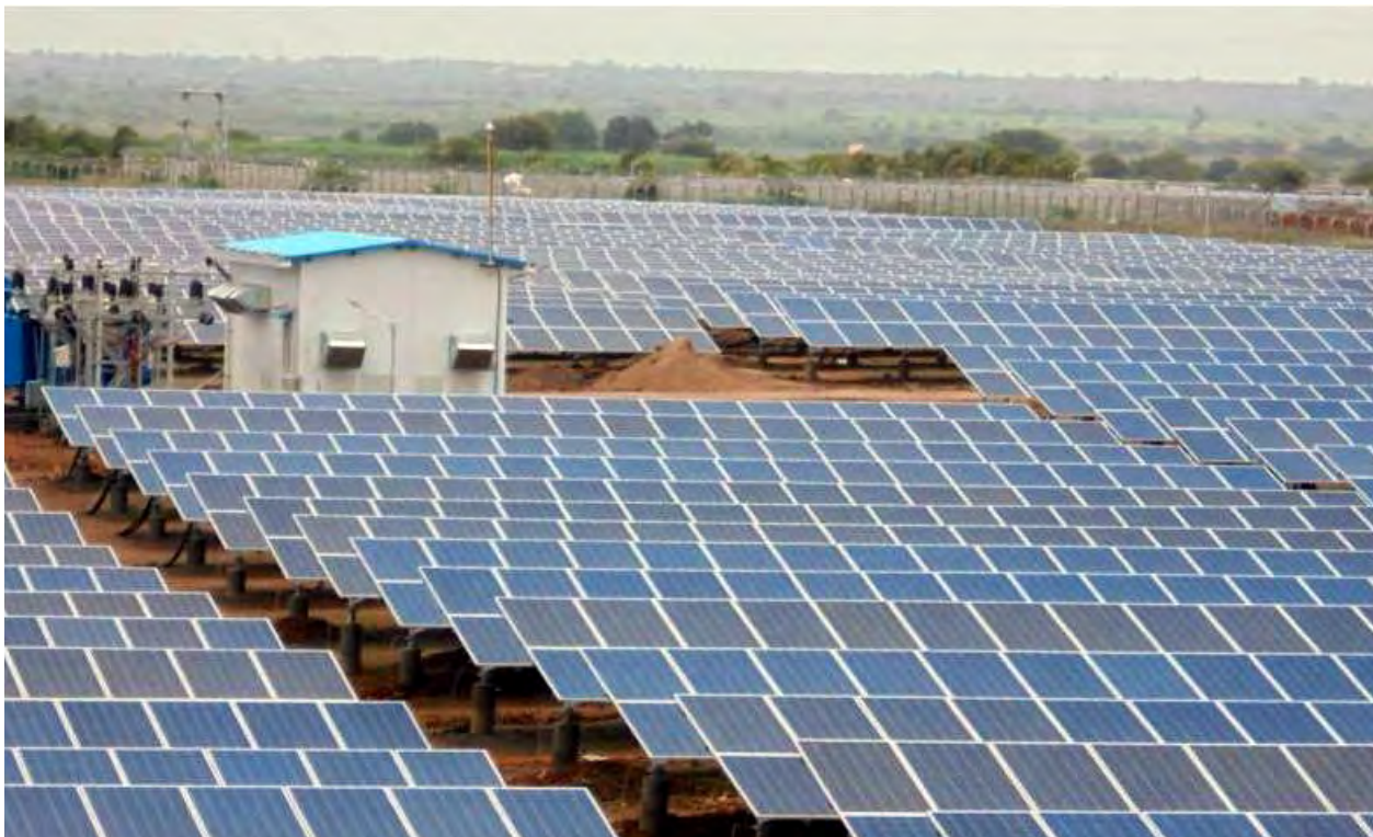
14MW Baramati Solar Power Plant
